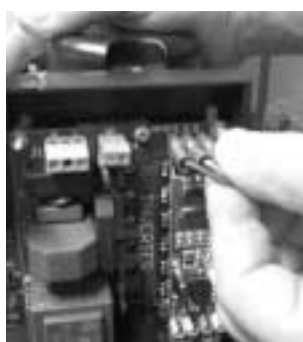
Motor cables on the inverter
