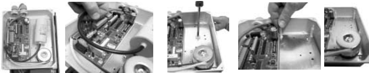
Detach and remove the capacitor
